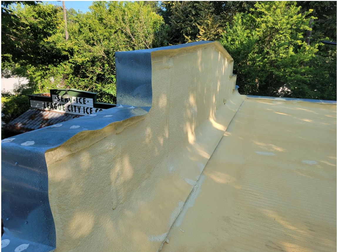
Spray expanding foam on roof and side / front walls (Continued on next page.)
